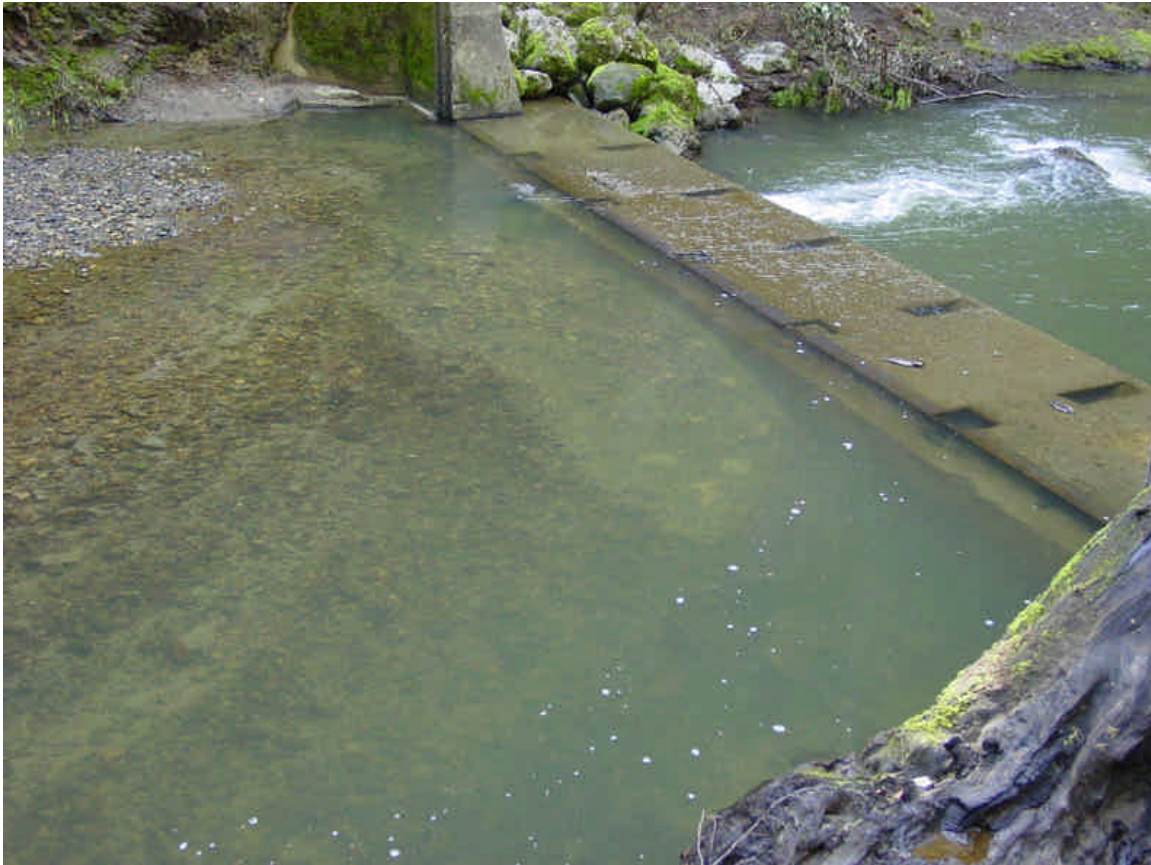
Figure 1. View of dam foundation from upstream. Large area of disturbed gravel at upper edge of foundation is steelhead redd. Chute through foundation is visible at upper right.
